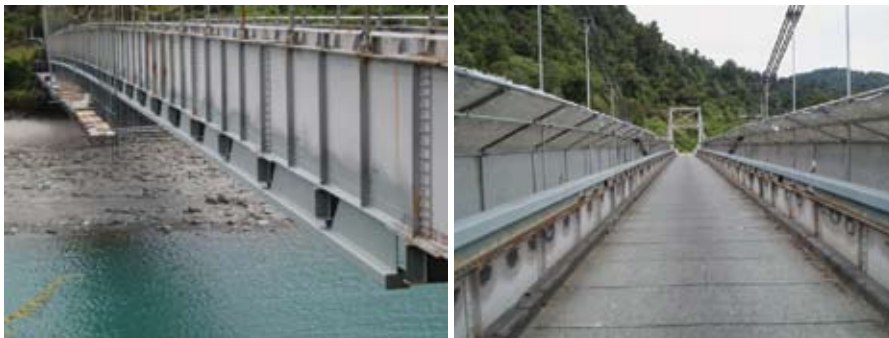
Karangarua Bridge which is now complete. The work carried out means that the bridges have new and longer steel support beams under them.
