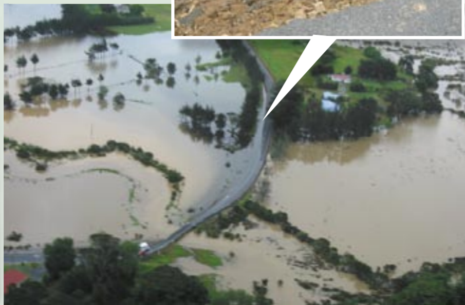
Widespread flooding in Northland (left) saw the Mitimiti Bridge (above) collapse.
